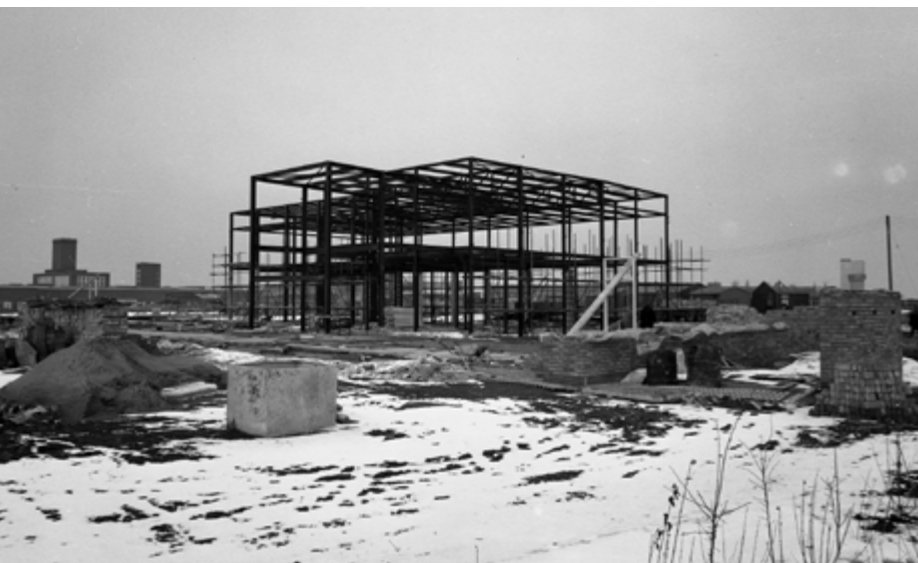
The Atlas Computer Laboratory under construction, looking north-east towards AERE Harwell, February 1963. The Tandem Van der Graaf Generator is just visible against the skyline on the far right of the photo.
