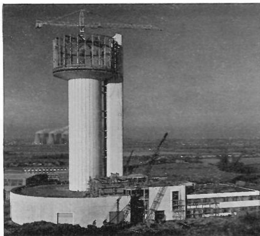
Picture (taken in December last year) shows the progress made on the Nuclear Structure Facility (NSF) at Daresbury
