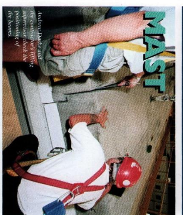
Harwell Defence and Nuclear Establishment staff are fitting a pre-cast concrete roof to the MAST fusion experiment.
