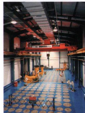
The interim radwaste store where canned waste is stored in a honeycomb of concrete lined holes.
