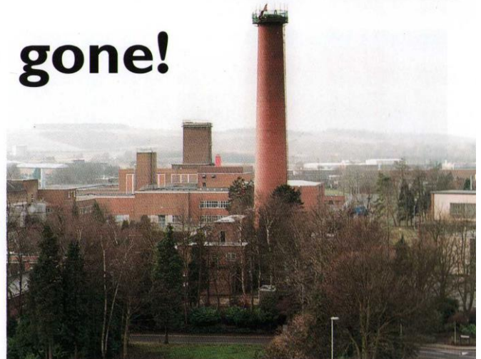
The Union Flag symbolises the 'detopping' in 2000. The scaffolding was lowered from the top, as the chimney shortened, and held in place by a clamping band.
