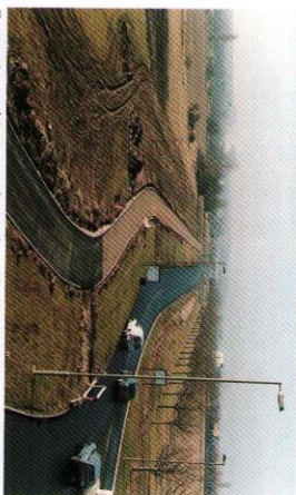
Construction work is now nearly complete. The principal contractor was Gordon Hill & Son, with trees provided and planted by CL.
