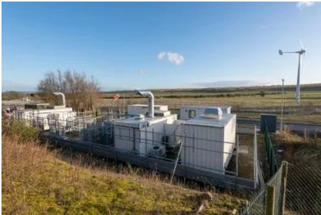
Green Ammonia Demonstrator.
