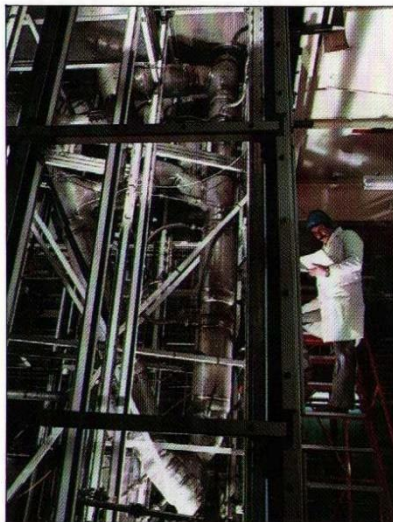
This experimental rig was constructed at Harwell in collaboration with the Nuclear Plant Design Office at the UKAEA's Risley Nuclear Power Development Establishment. The rig is a full-scale inactive prototype of a batch dissolver under development for the reprocessing of fuel from a Commercial Demonstration Fast Reactor.
