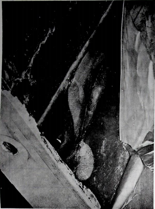
Fig. 8.7(ii) Crushing and voids on a vacuum vessel.
