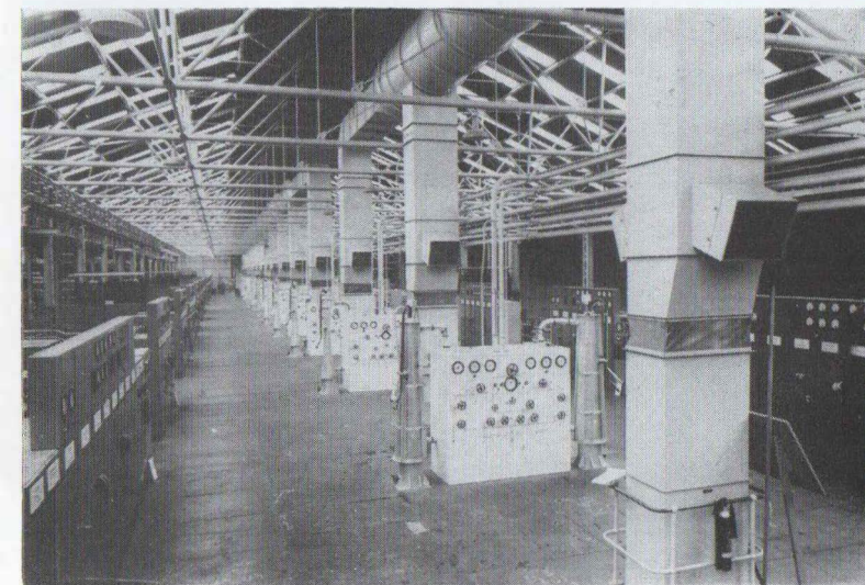
Operating Platform — Capenhurst
